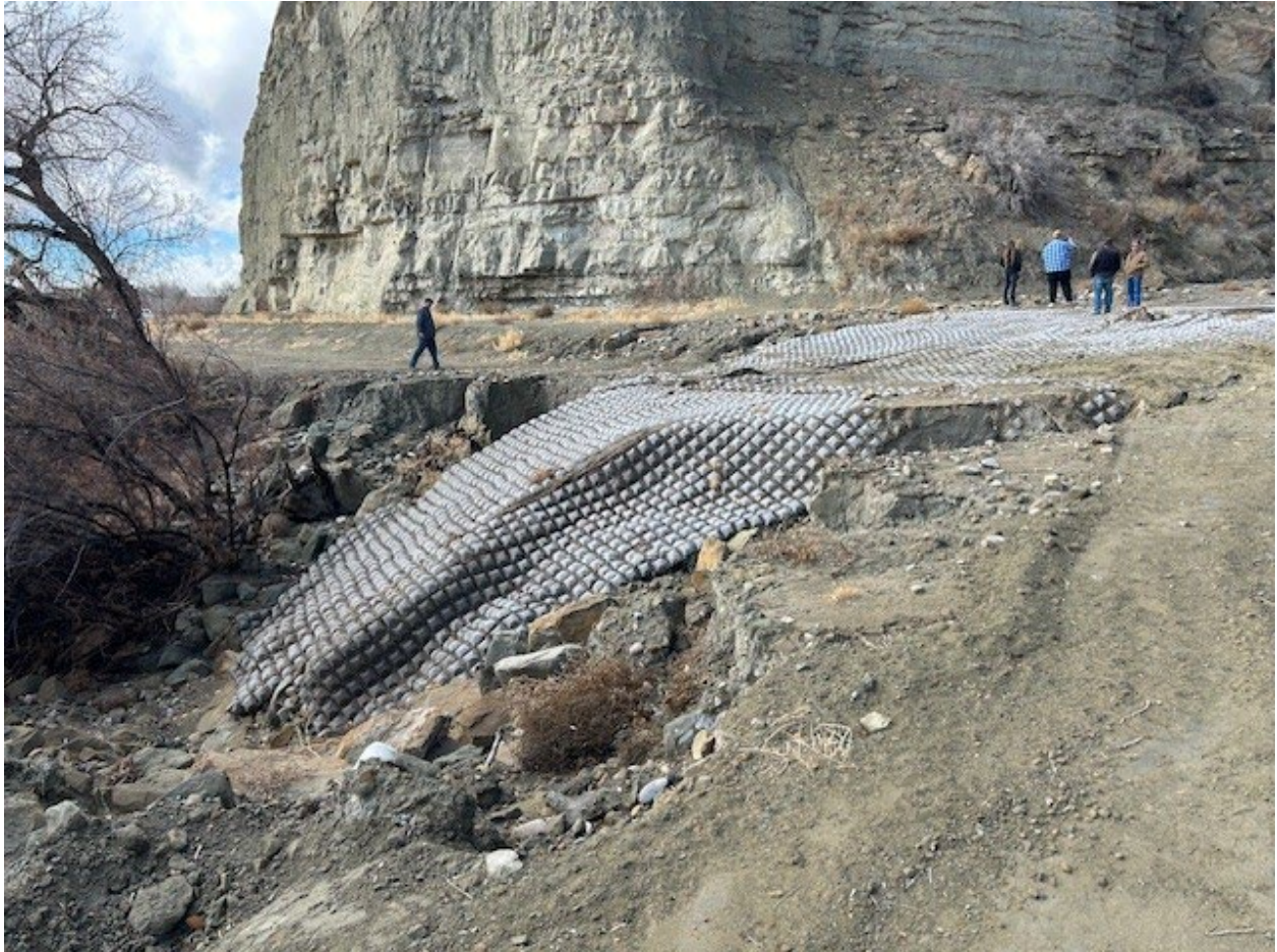
Figure 3. Erosion of the Access Road
