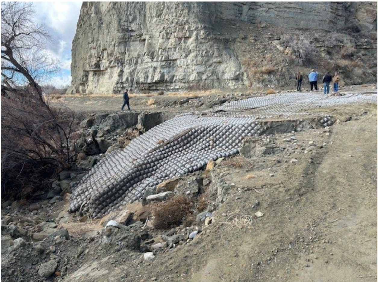
Figure 3. Erosion of the Access Road
