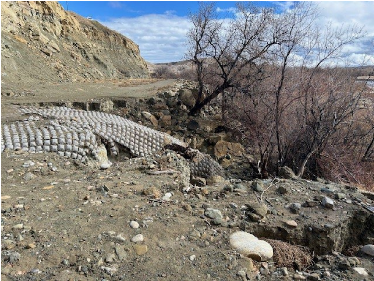
Figure 1. Erosion of the Access Road.
