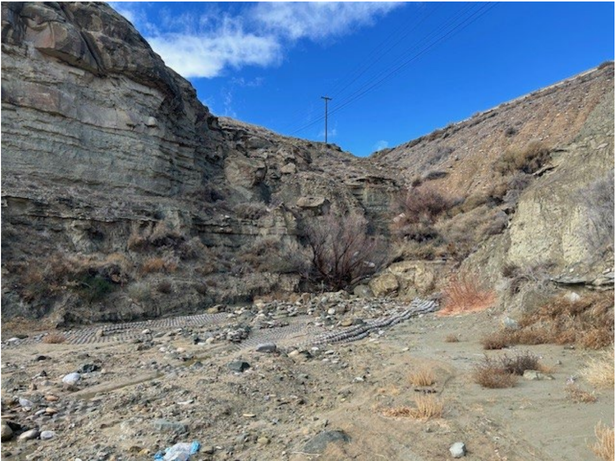
Figure 4. Damage to the ACB Matting
