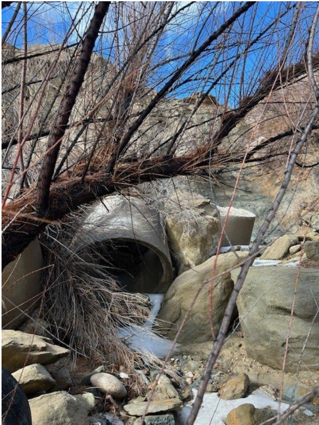
Figure 5. Pieces of the Culvert that was Installed Upslope
